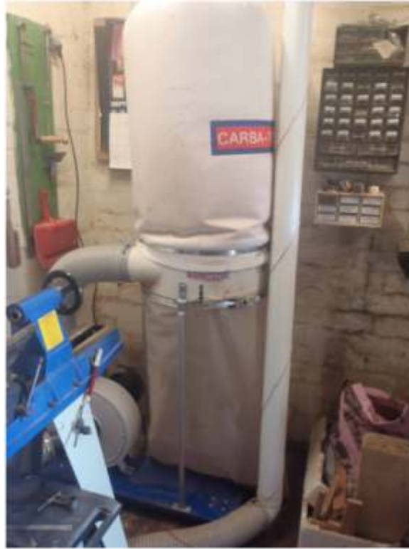
NEW DUST EXTRACTOR WITH SOME OF THE PIPES
